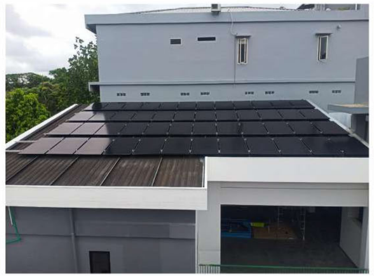
@ Ambon - 15 kW On Grid
