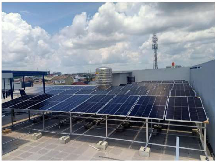
@ Palembang - 30 kW On Grid
