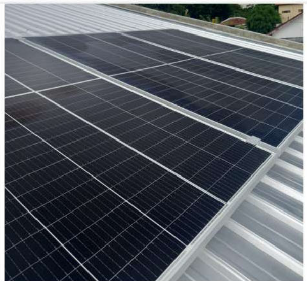
@ Klaten - 5 kW On Grid
