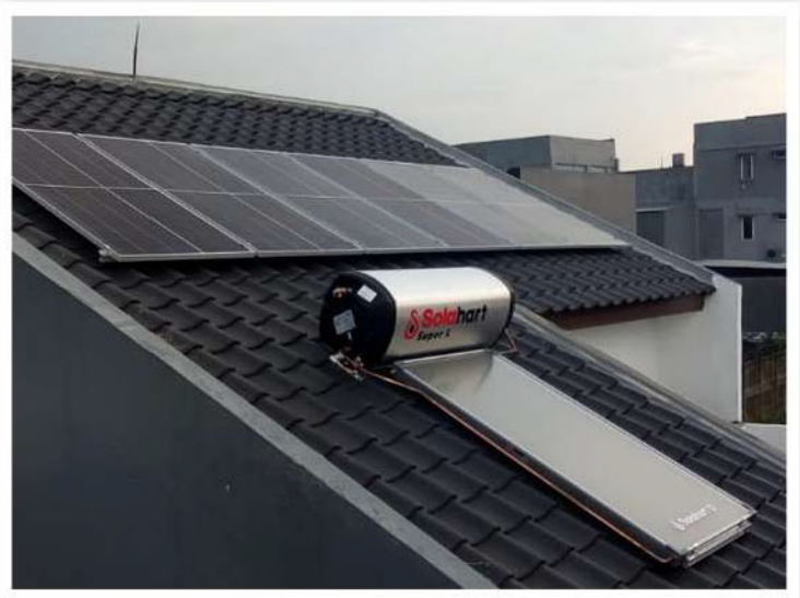
@ Bintaro - 3 kW On Grid
