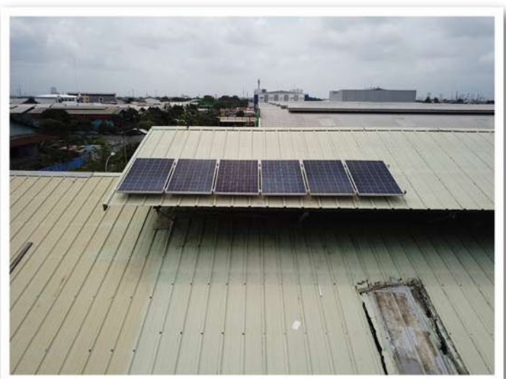
@ Daanmogot - 1 kW On Grid
