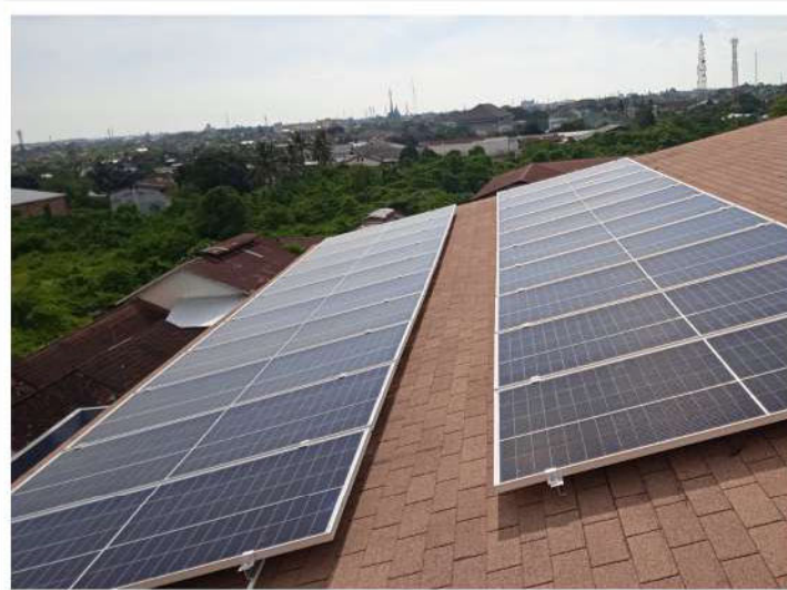
@ Lombok - 10 kW On Grid
